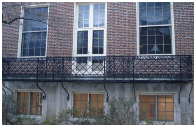
Figure 4: Balconies raise new concerns.
